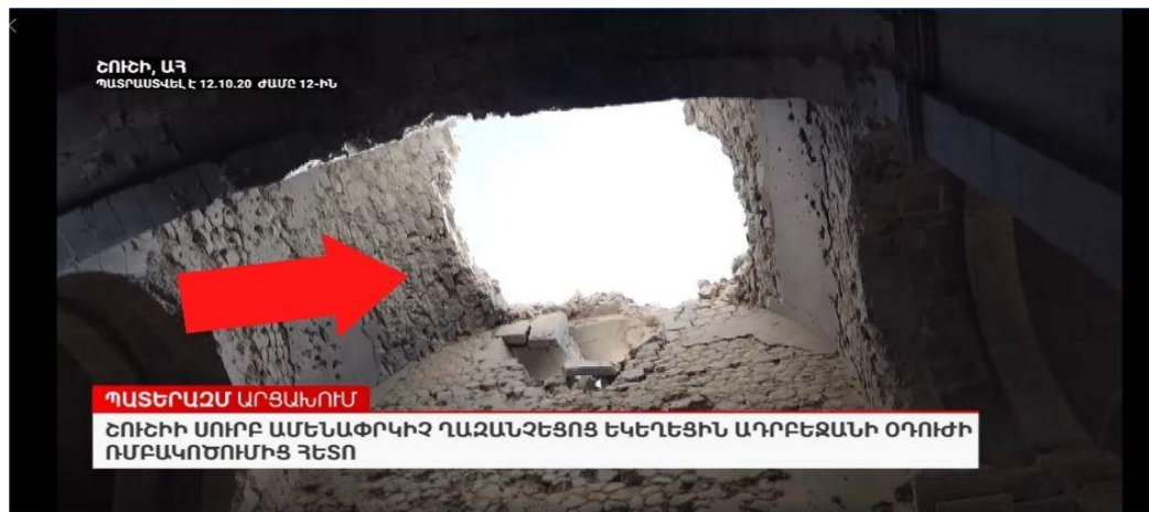
Picture 6. The damaged roof of the St. Holy Savior Ghazanchetsots Cathedral from inside after the second strike
